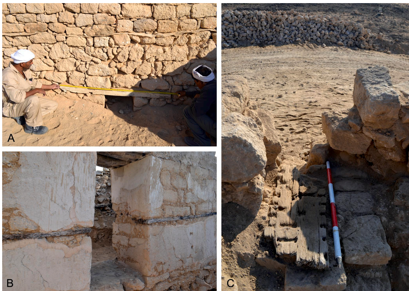
Fig. 3. (A): A ship beam recycled as a lintel over a small window. (B and C): Ship planks used as levelling courses in the walls of the al-Balid citadel. (Photos: A. Ghidoni).
