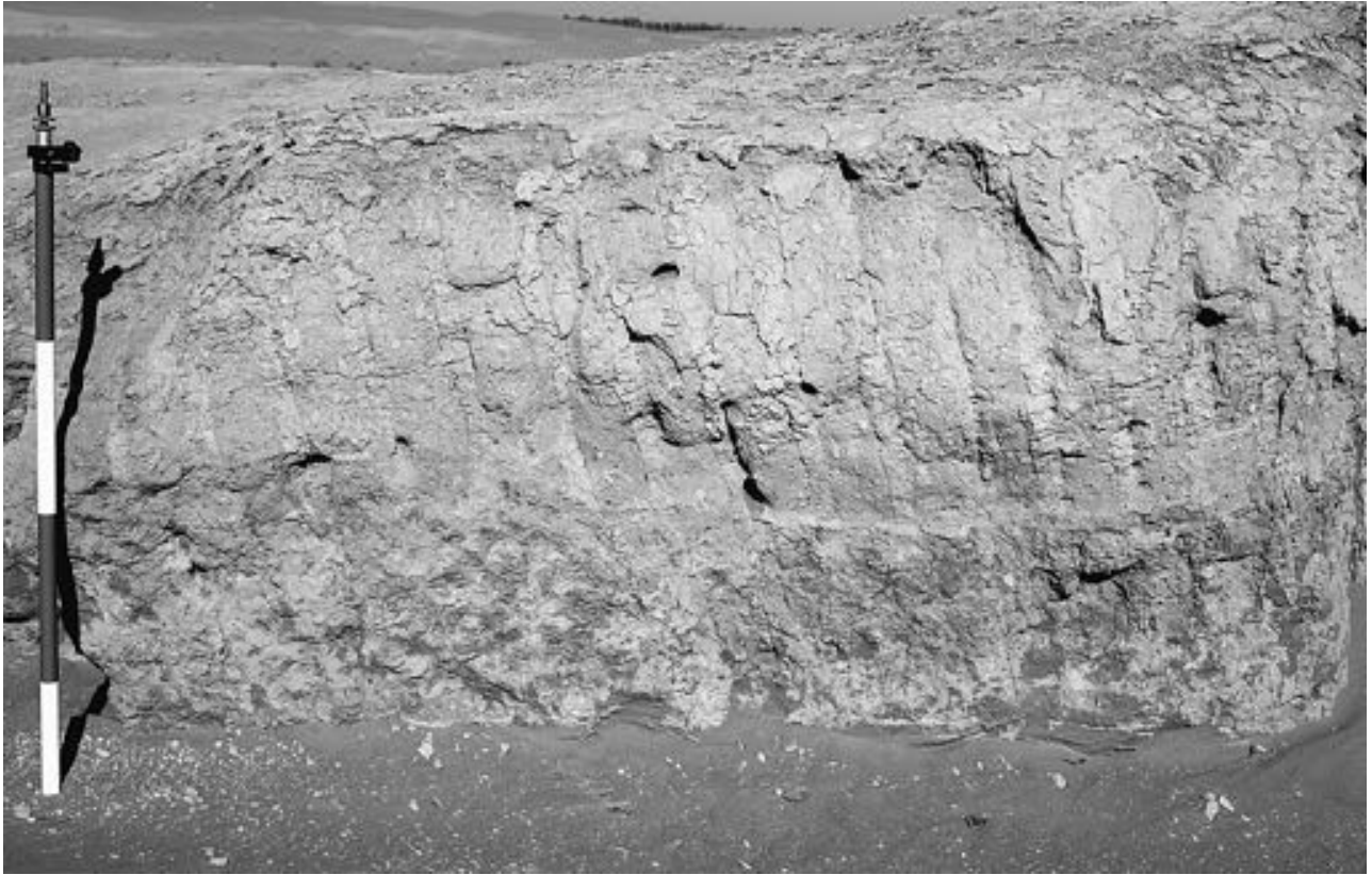
Fig. 11. Detail of the "pitched" mud-brick work of the main vault (western plinth).
