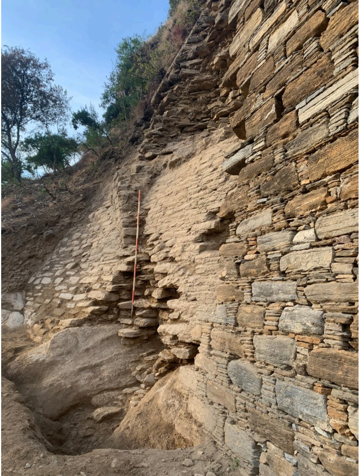
Fig. 15. Overlay of the masonry phases of the east corner (IAMP, CC BY-NC-ND 4.0)
