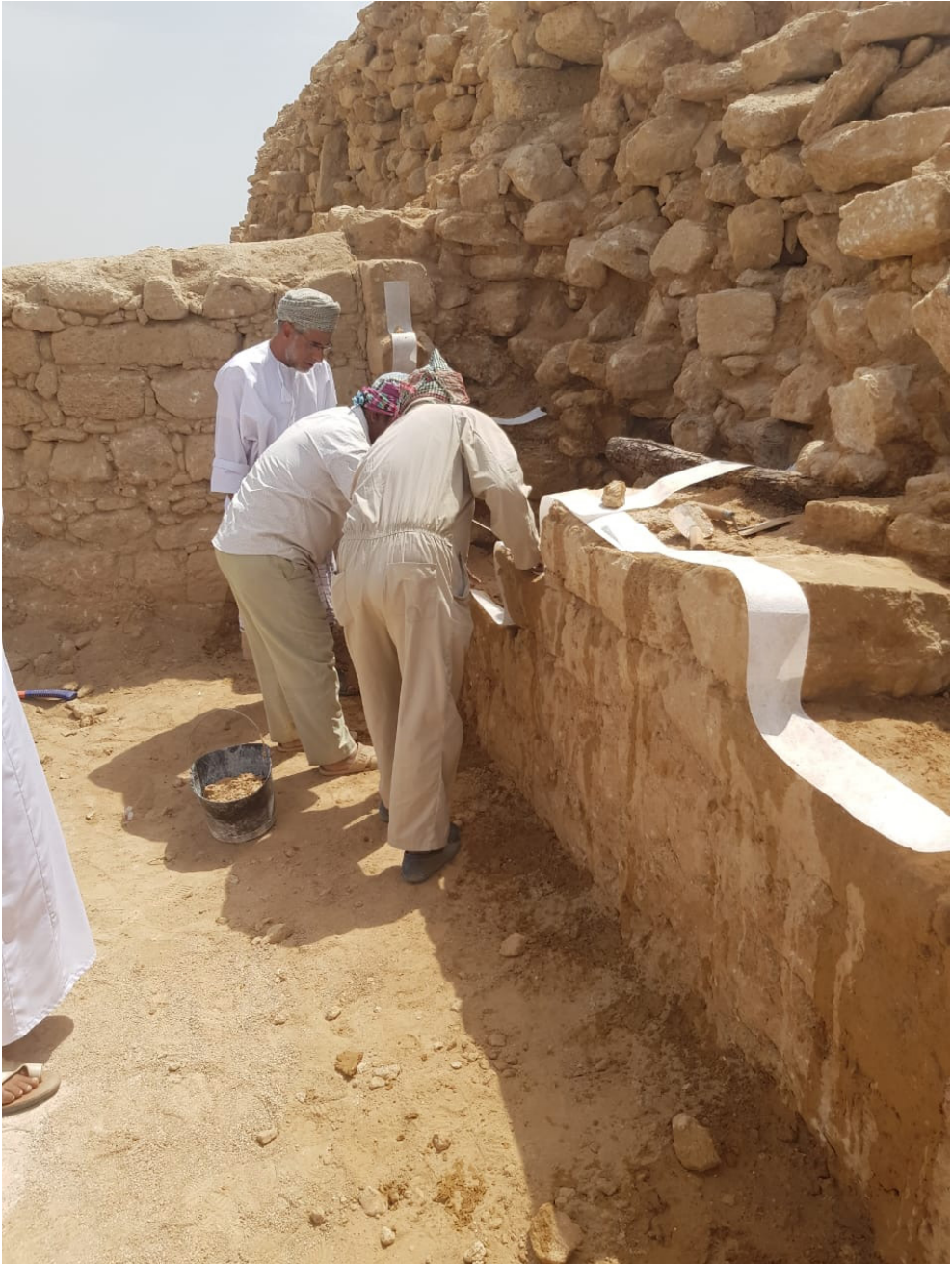
Fig. 5. Restoration works at the site (© Italian Archaeological Mission of L'Orientale at Al Baleed)
