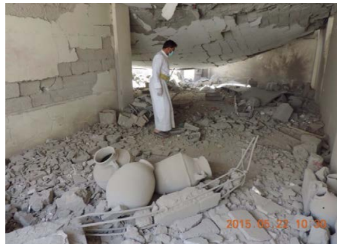
Figure 2: Dhamar Regional Museum on the day of its destruction, both in May 2015. Source: UNESCO
