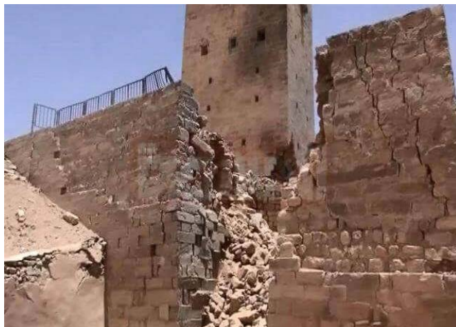
Figure 1: Marib Dam, after the bombing in May 2015 Source: UNESCO
