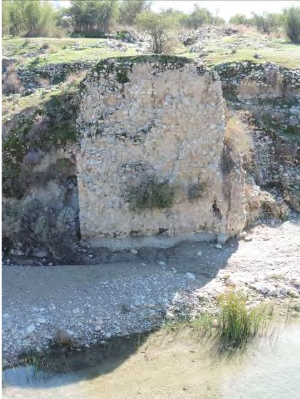
Fig. 5 - The western pilon of the bridge Pol-e Gabrī, as seen from right bank of the river, after MAI
