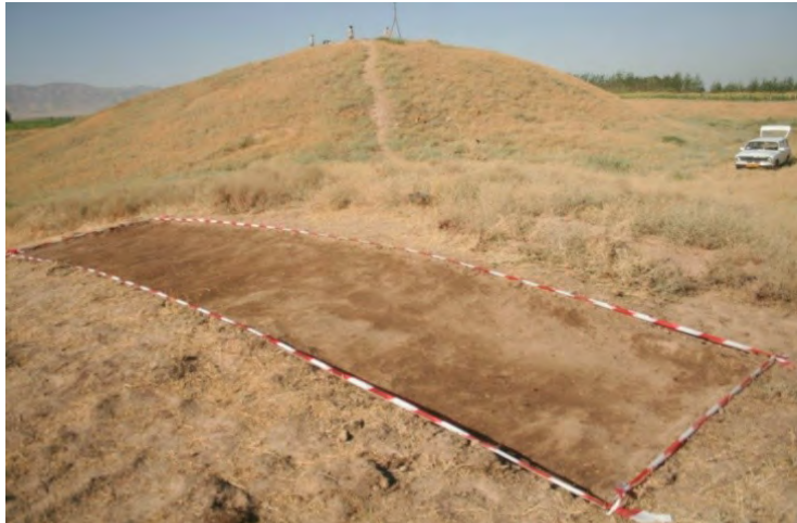
Fig. 26 - Trench no 9 after the 1st cutting as seen as from North-East, MAI, after B. Genito
