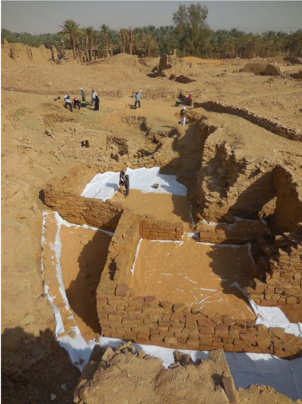
Fig. 10 - Final protective step, placement of the cover non-woven Geodren 200. View from South
