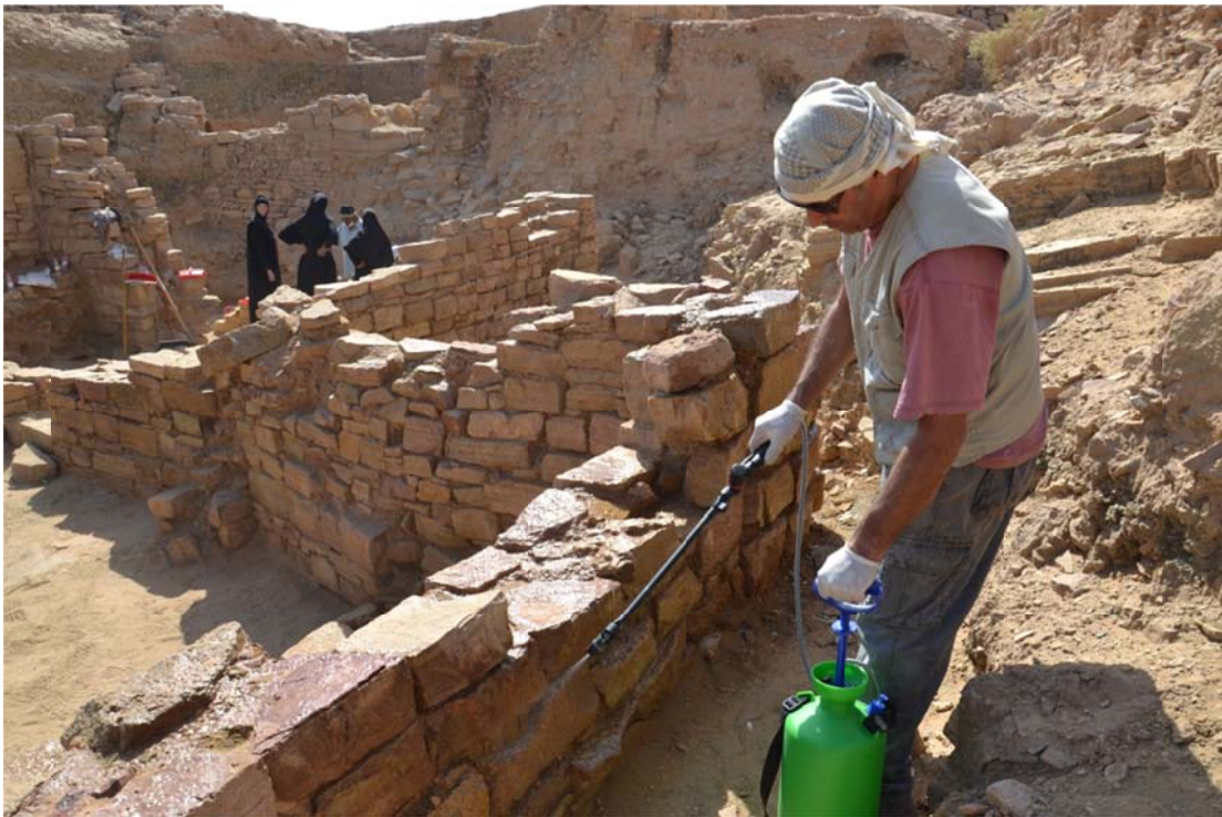
Fig. 7 - Detail of the consolidation of the façade of the Building A walls
